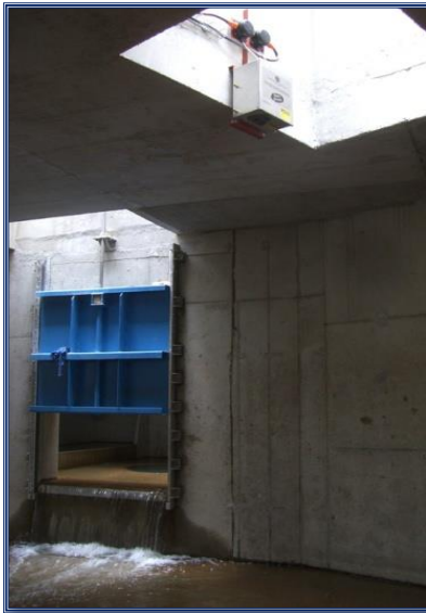
Underground Effluent Discharge Monitoring Application
